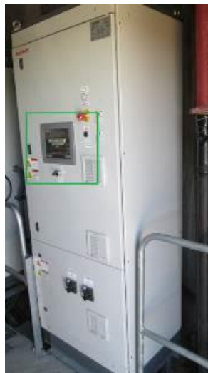
Armario ground Controller, resaltado en verde la pantalla y el selector de apagado / encendido. Ground control cabinet, with the screen and ON/OFF selector outlined in green.
